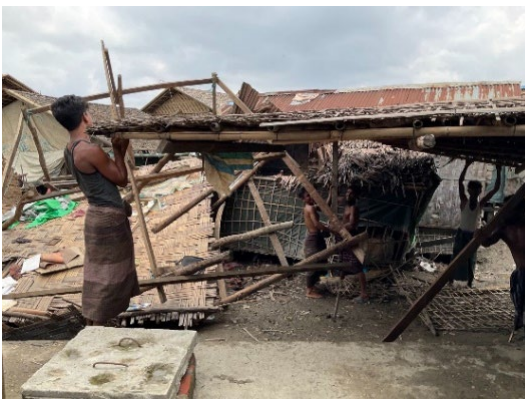
A shelter damaged by Cyclone Mocha that is being repaired in Nget Chaung 2 IDP camp. Pauktaw, Rakhine. Credit: OCHA
