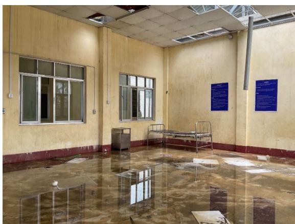
Thet Kae Pyin Station Hospital is out of action following damage from Cyclone Mocha. Sittwe. Rakhine. Credit: OCHA
